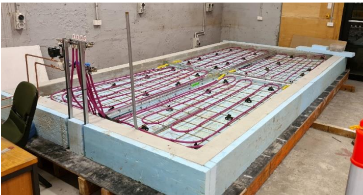
Figure 23: Heated slab with insulated forma, and hydronic heating coils attached to the reinforcement.
