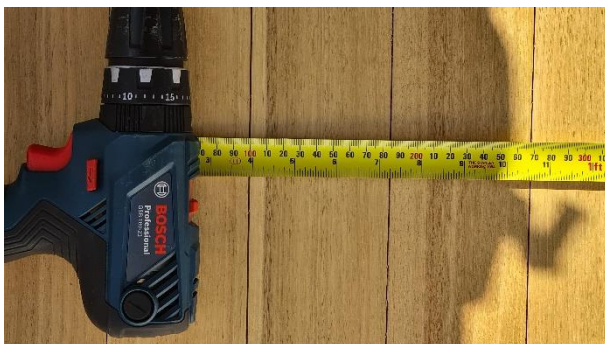
Regular gapping in floor
