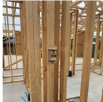
Figure 15: Sensor-only unit on a timber frame.
