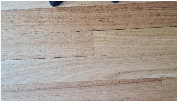
Figure 3: Minor slabbing from board adhesion.
