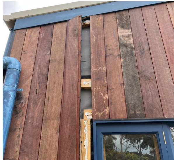
Figure 10: Board removed to relieve expansion pressure.
