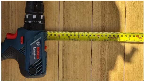
Figure 4: Regular gapping in floor
